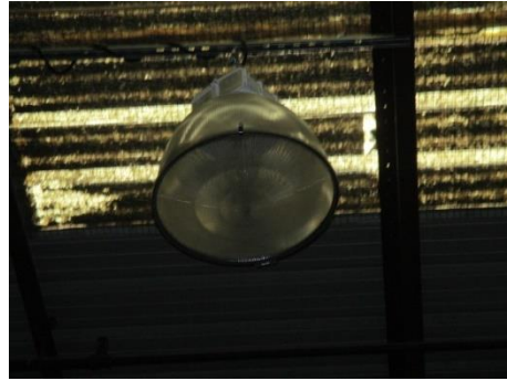
Mercury vapor light in the warehouse.
