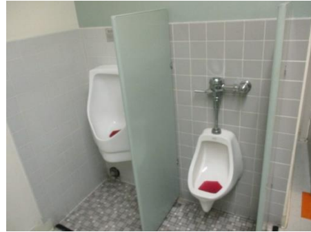
Lead-laden ceramic wall trim in the men's bathroom behind and next to urinals
