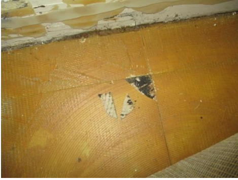
Asbestos containing black floor mastic and floor tile contaminated with the mastic.
