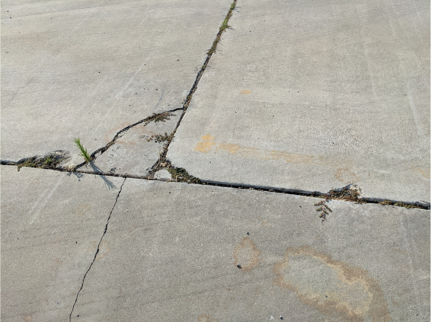
Image 3 – Typical Corner Break on Slab
