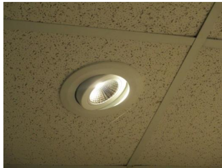
Unidentified light type inside the subject property building.
