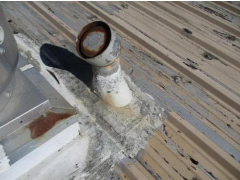
Asbestos containing transite flue on roof.
