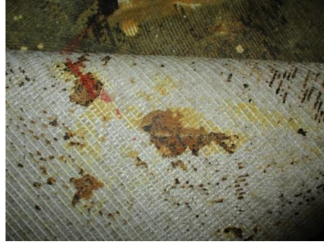
Asbestos containing black floor mastic and carpeting contaminated with the mastic.
