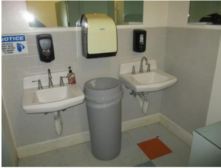
Lead-laden ceramic wall trim in the men's bathroom behind and next to sinks.
