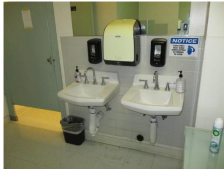
Lead-laden ceramic wall trim in the woman's bathroom behind and next to sinks.
