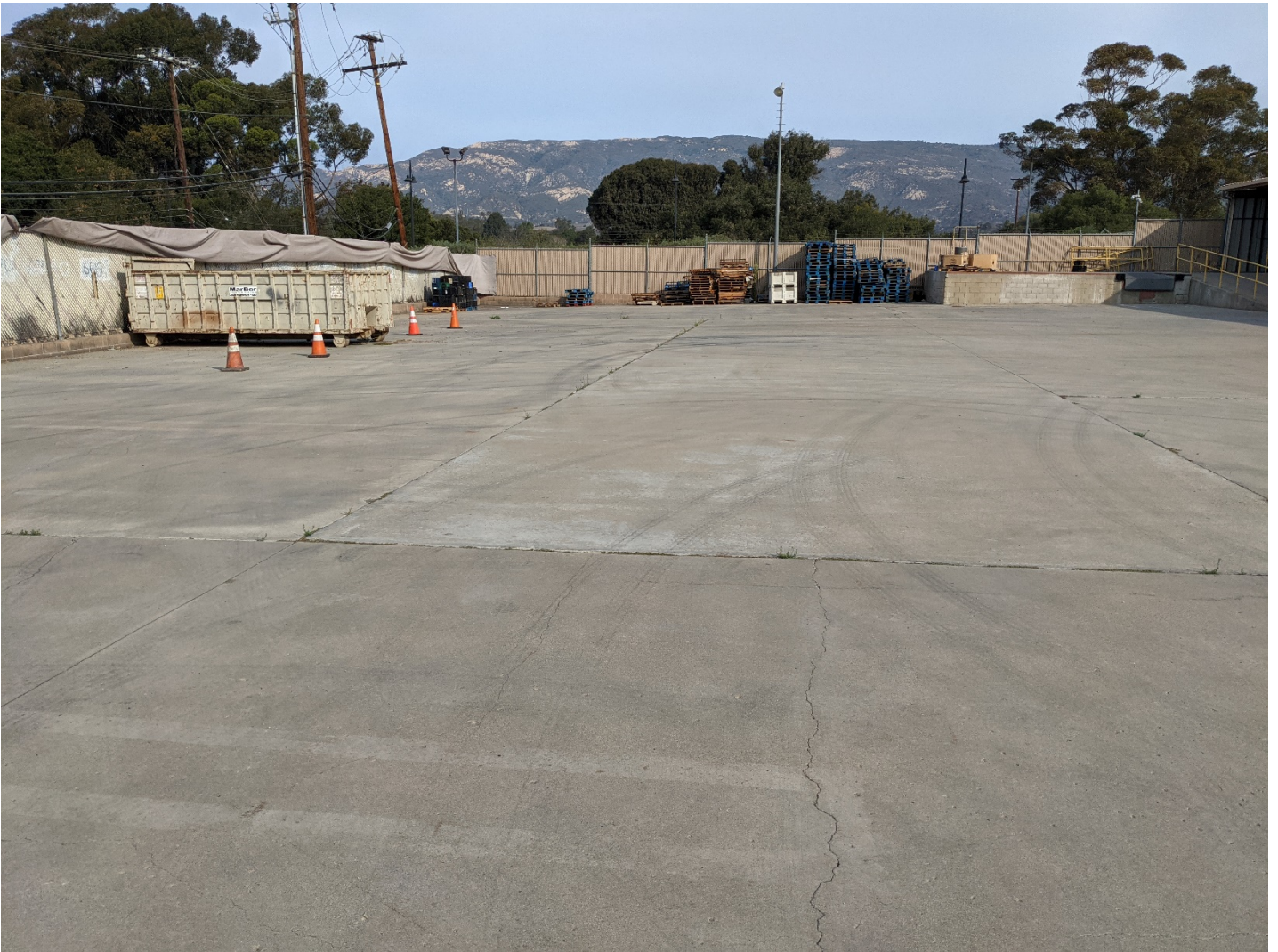
Image 1 – General Site View Showing Typical Mid-Slab Cracking
