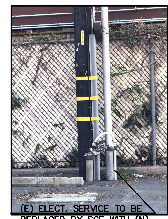
3 ELECTRICAL POC REFERENCE IMAGE #3
