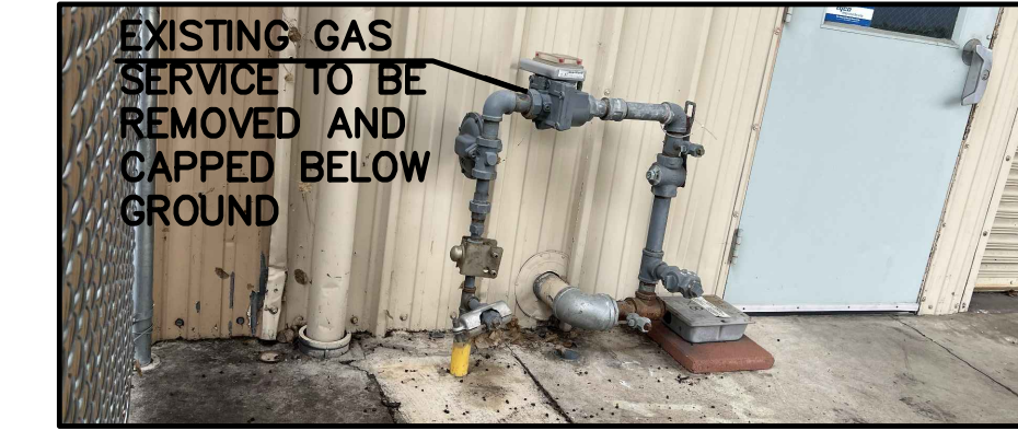
5 EXISTING GAS METER REFERENCE IMAGE #5
