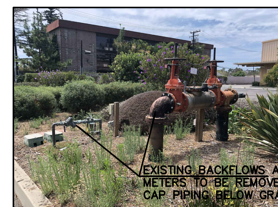
6 EXISTING METERS / BACKFLOWS REFERENCE IMAGE #6
