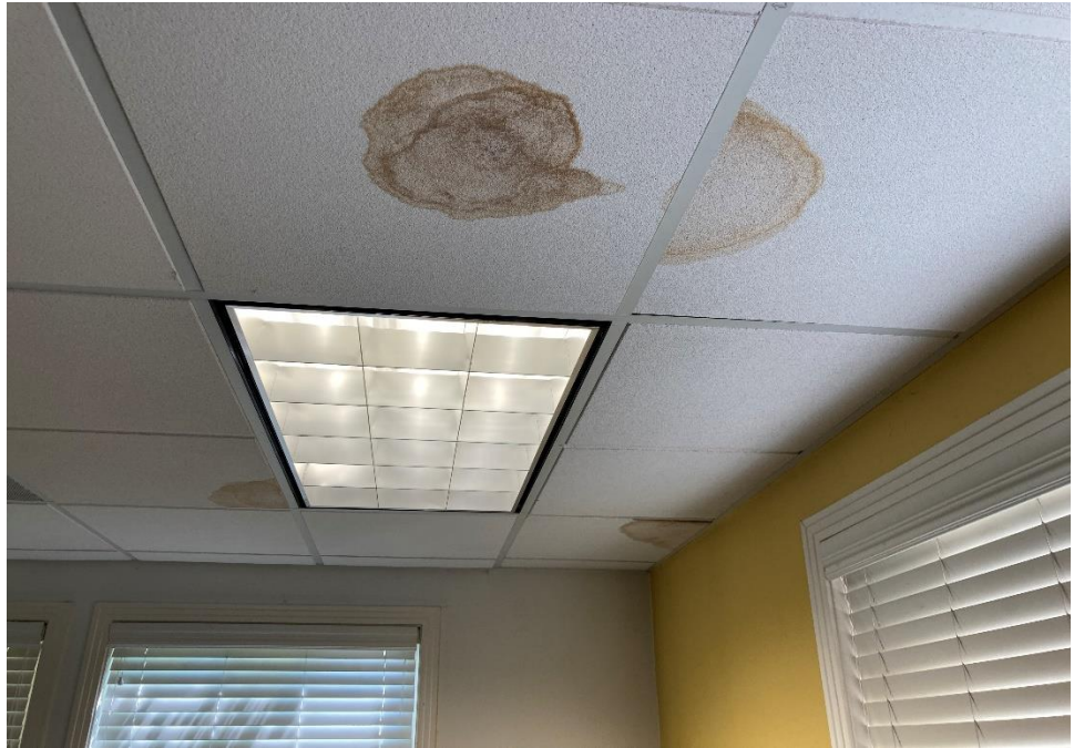
Photograph 9: Representative view of the water damage in the Storage room.
