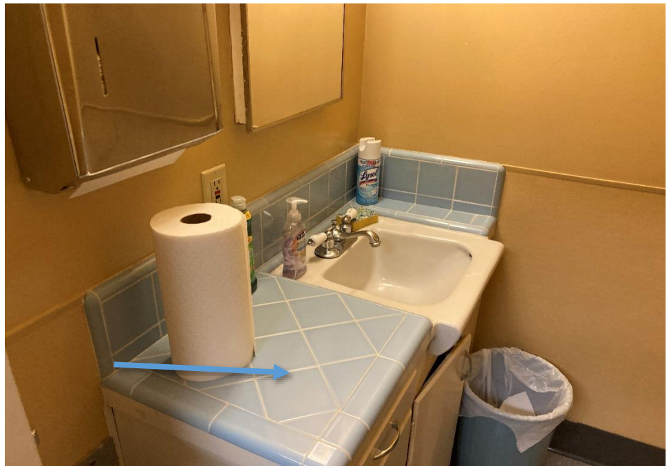
Photograph 8: View of the lead containing ceramic countertop in Restroom 1.
