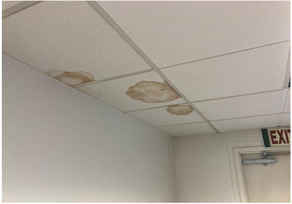
Photograph 11: Representative view of water damage in Office 6.
