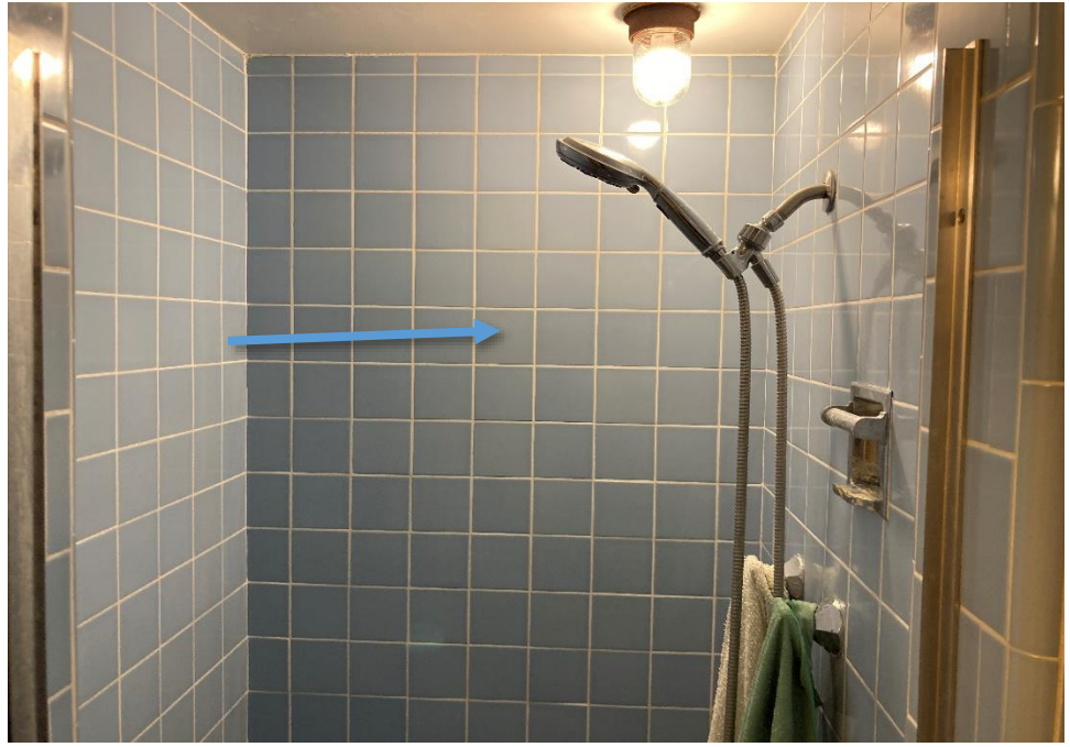
Photograph 7: View of the lead containing blue ceramic tile in Restroom 1.
