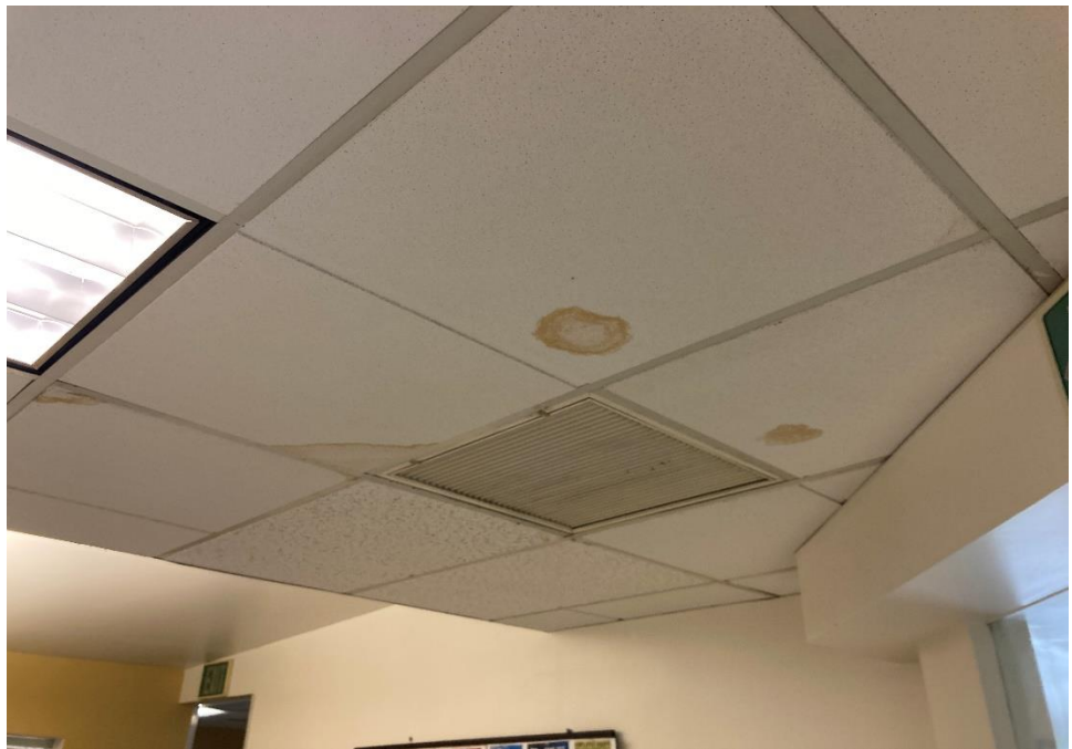
Photograph 10: Representative view of the water damage in Lobby 1.
